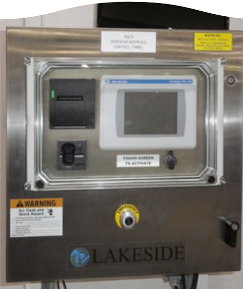
RACS Control Panel
