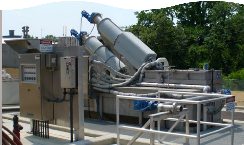
Septage Complete Plant with Electrical Control Panel
