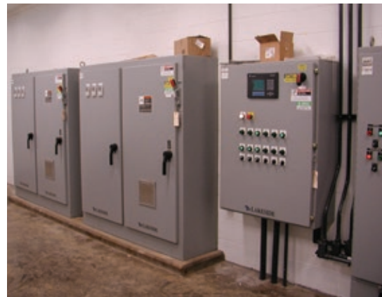
Programmable Logic Controller (PLC) Based System
