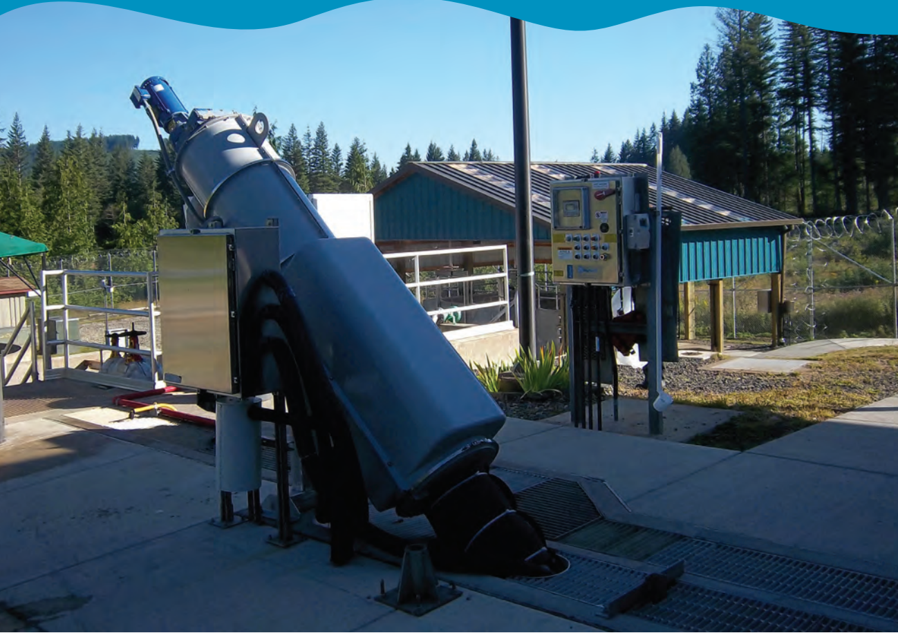
YACOLT, WASHINGTON LARCH CORRECTIONS CENTER WWTF
