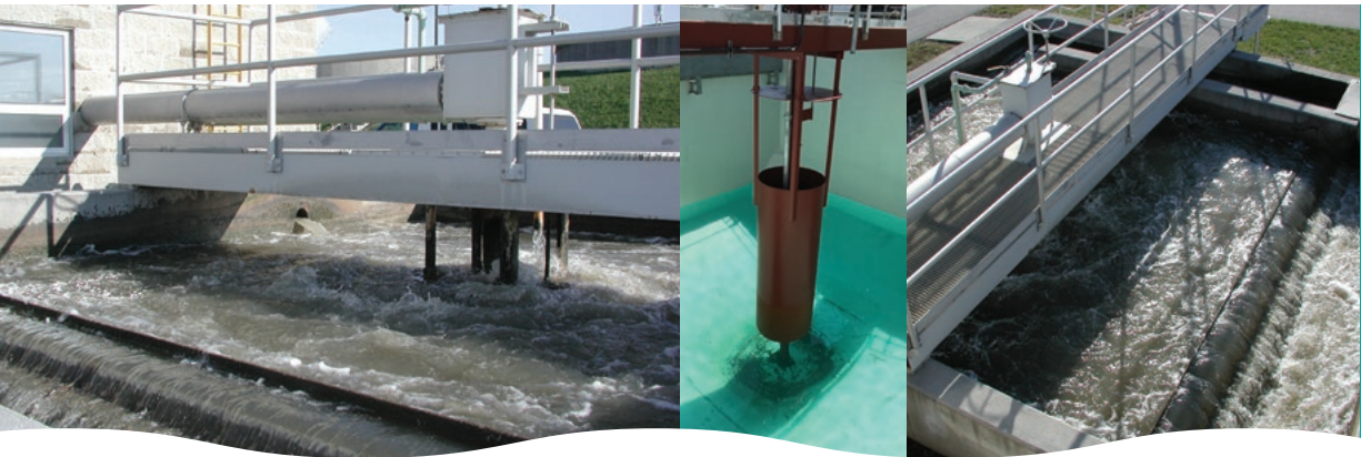
Aeroductor Grit Removal System
