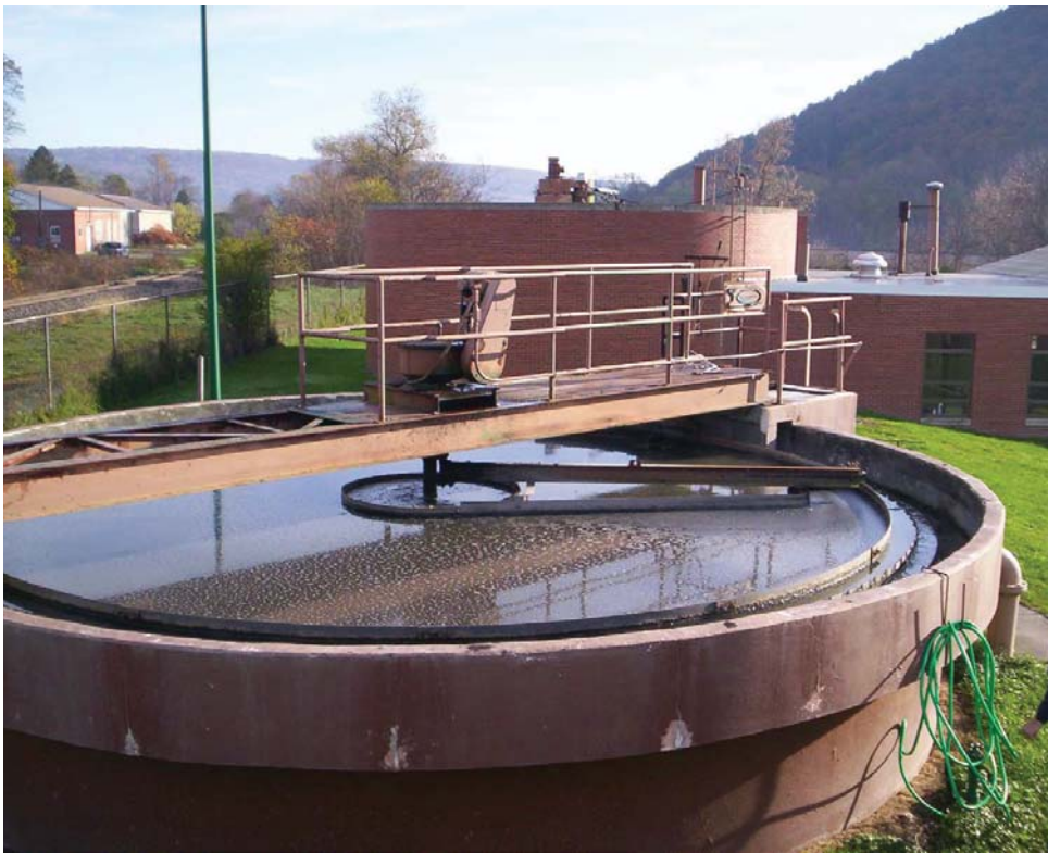
CLARIFIER PRE-CONSTRUCTION AT ADDISON, WORN GEARBOX, CRACKED WALLS AND A WORN ARM THAT WOULD OFTEN STICK
