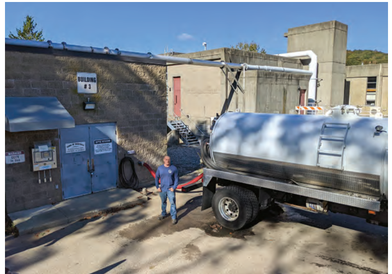
Operator Scott Farrington with the Septage Acceptance Plant at the Montville clean-water facility.
