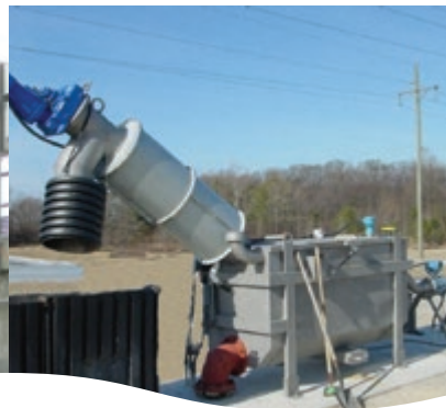
Raptor® Septage Acceptance Plant
