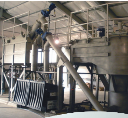
Horizontal and Grit Dewatering Screws
