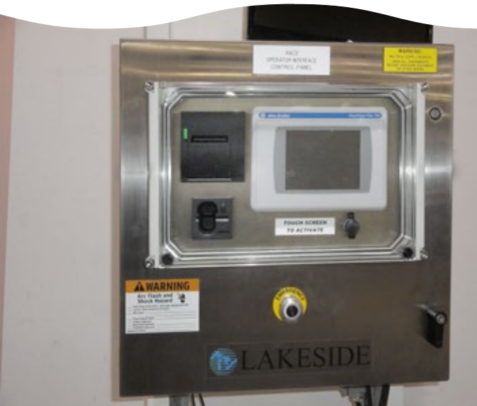
RACS Control Panel
