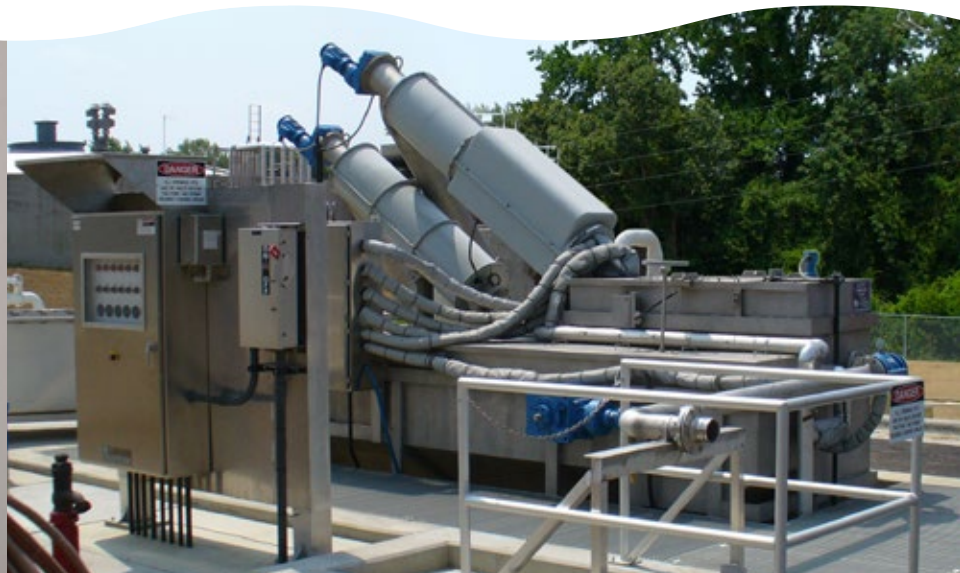
Septage Complete Plant with Electrical Control Panel
